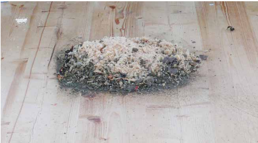
Waste from one week during the erection of the CLT frame at Stadhaus/Murray Grove
